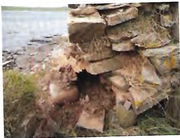
Recent gale damage
